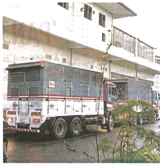
Sabah Electricity Sdn Bhd (SESB) mobile generator sets supplying power to Hospital Queen Elizabeth in Kota Kinabalu yesterday. PIC COURTESY OF SESB
